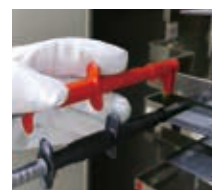
For clamping around the target busbar
