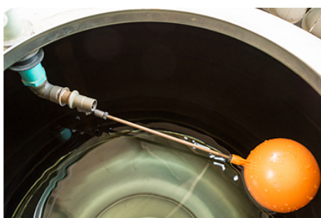
Level control float switch
