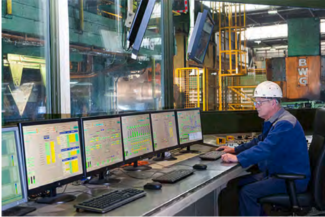
Reference: V7 control room
