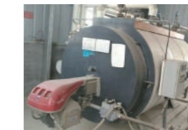
■ Air supply fan for boiler
